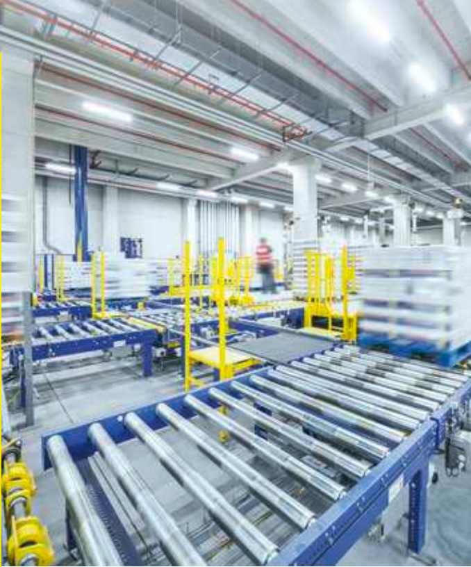
Roughly 2.6 km of conveying system for economical transport
