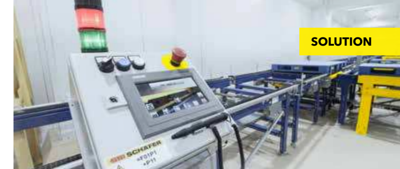
Monitors the inbound and outbound goods using WAMAS®
