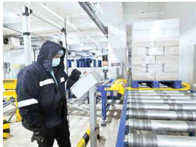
Pallets are transferred from a -18°C environment to the automated high-bay warehouse via conveyors
