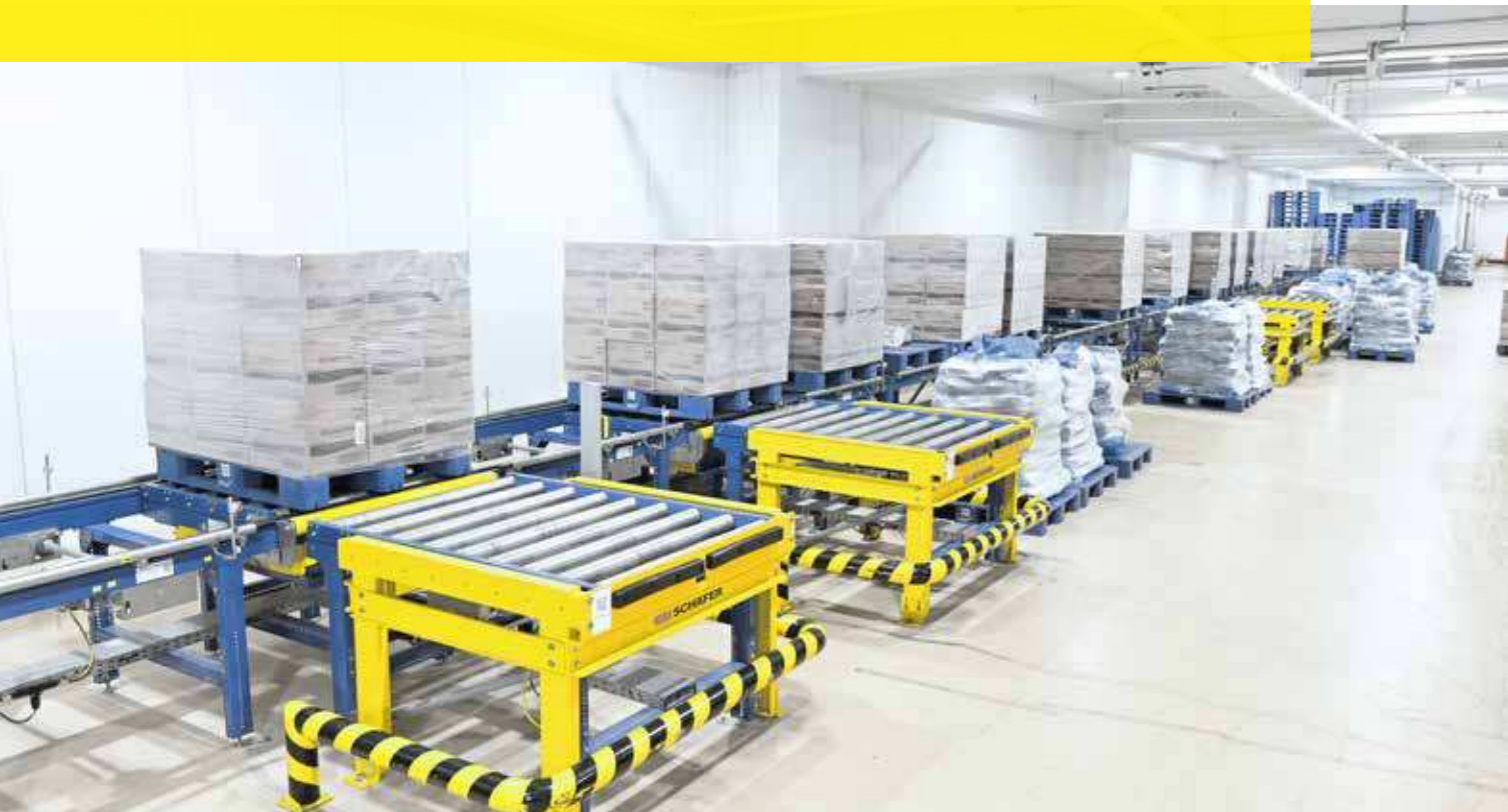
The 282 meters long conveying system connecting to key individual areas of the warehouse
