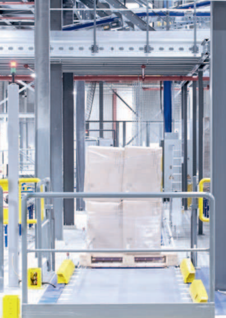
Transport of supplied goods to the high-bay warehouse
