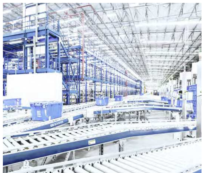
Carton and bin conveying system: avg. 28,900 bins throughput / day
