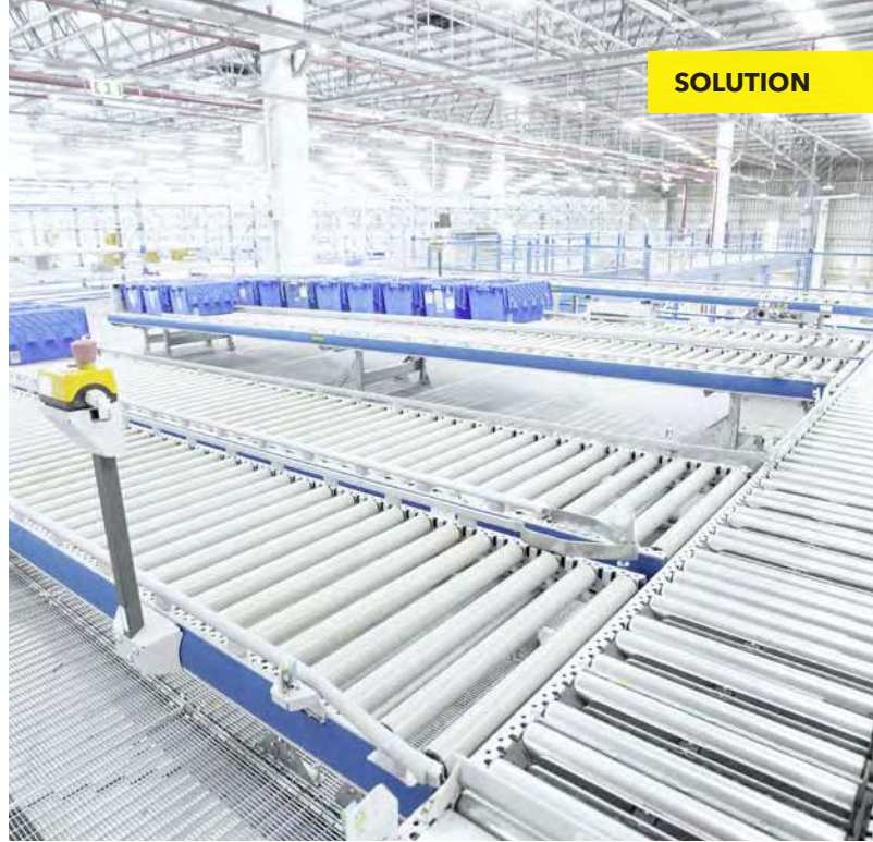
Carton and bin conveying system in connection with picking stations at the 3rd floor
