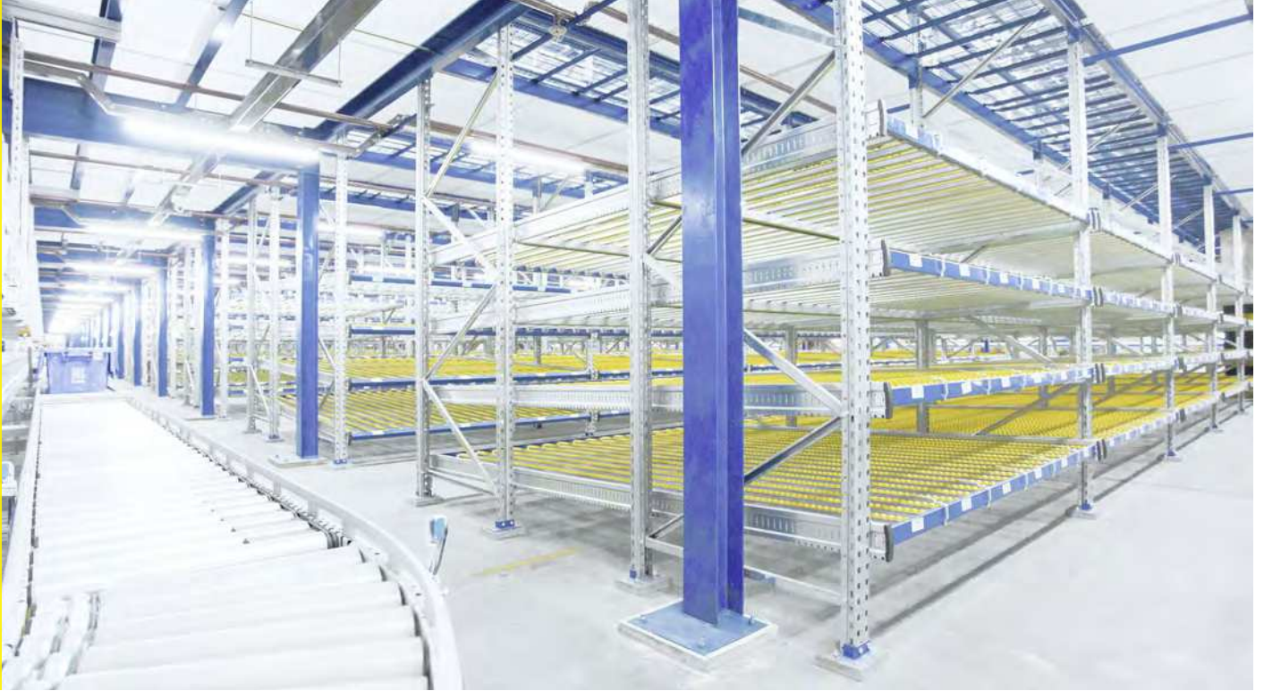
Carton flow racks at the ground floor are designed for faster-moving items and quicker replenishment
