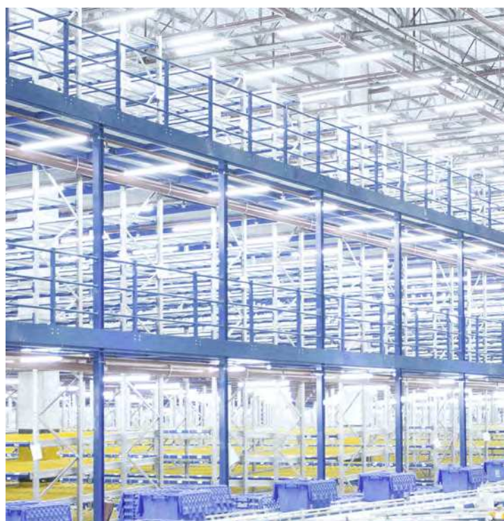
Carton flow racks and long-span shelvings as the mezzanine support system
