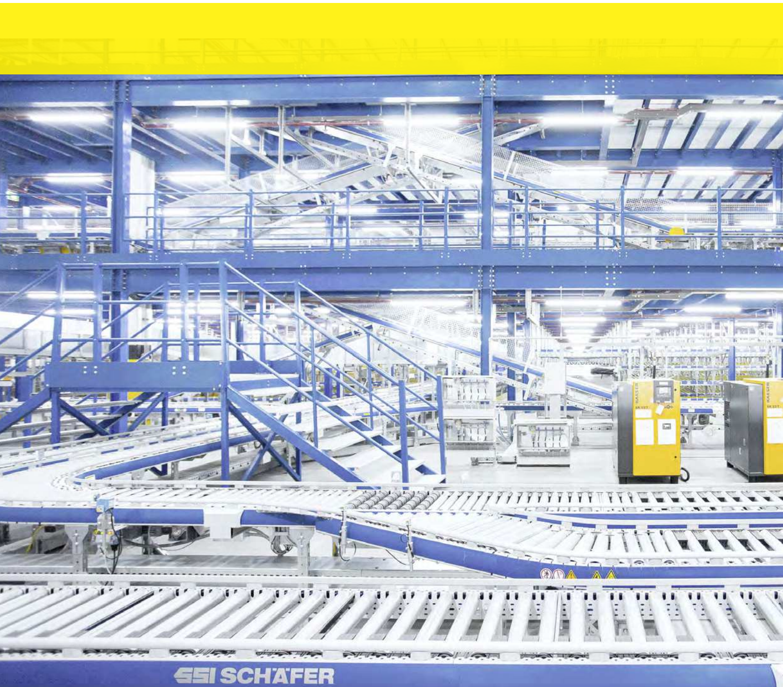
973 meters of carton and bin conveying system connecting to key individual areas of the warehouse
