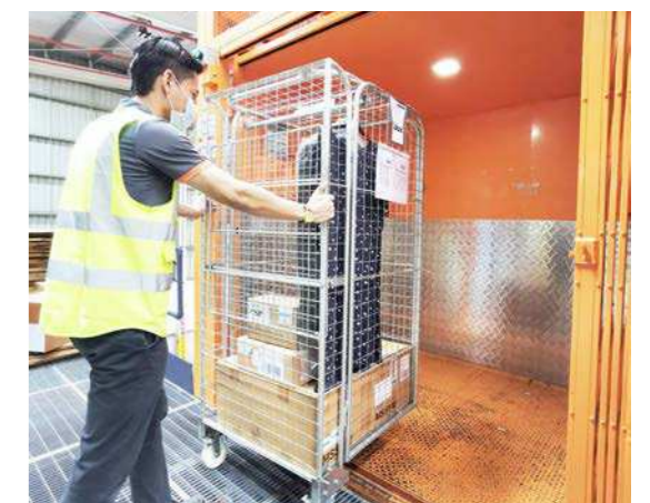
Cargo hoist for goods transfer between mezzanine floors
