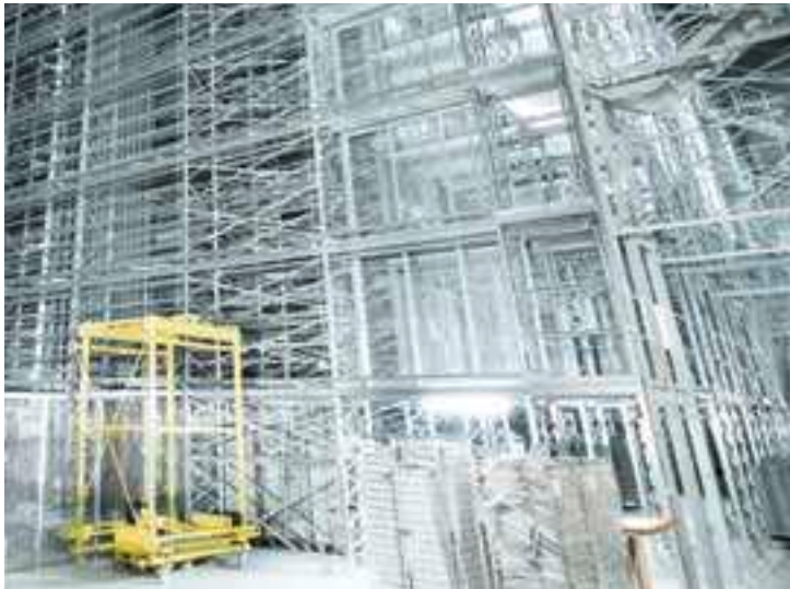
Shuttle area with 130,500 bin storage locations
