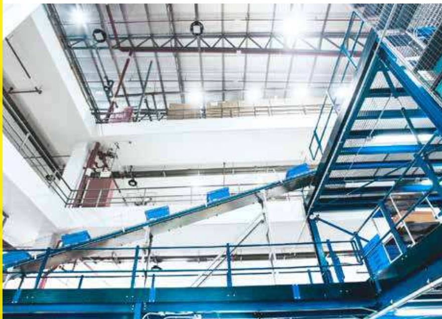
Carton and bin conveying system for economical transport
