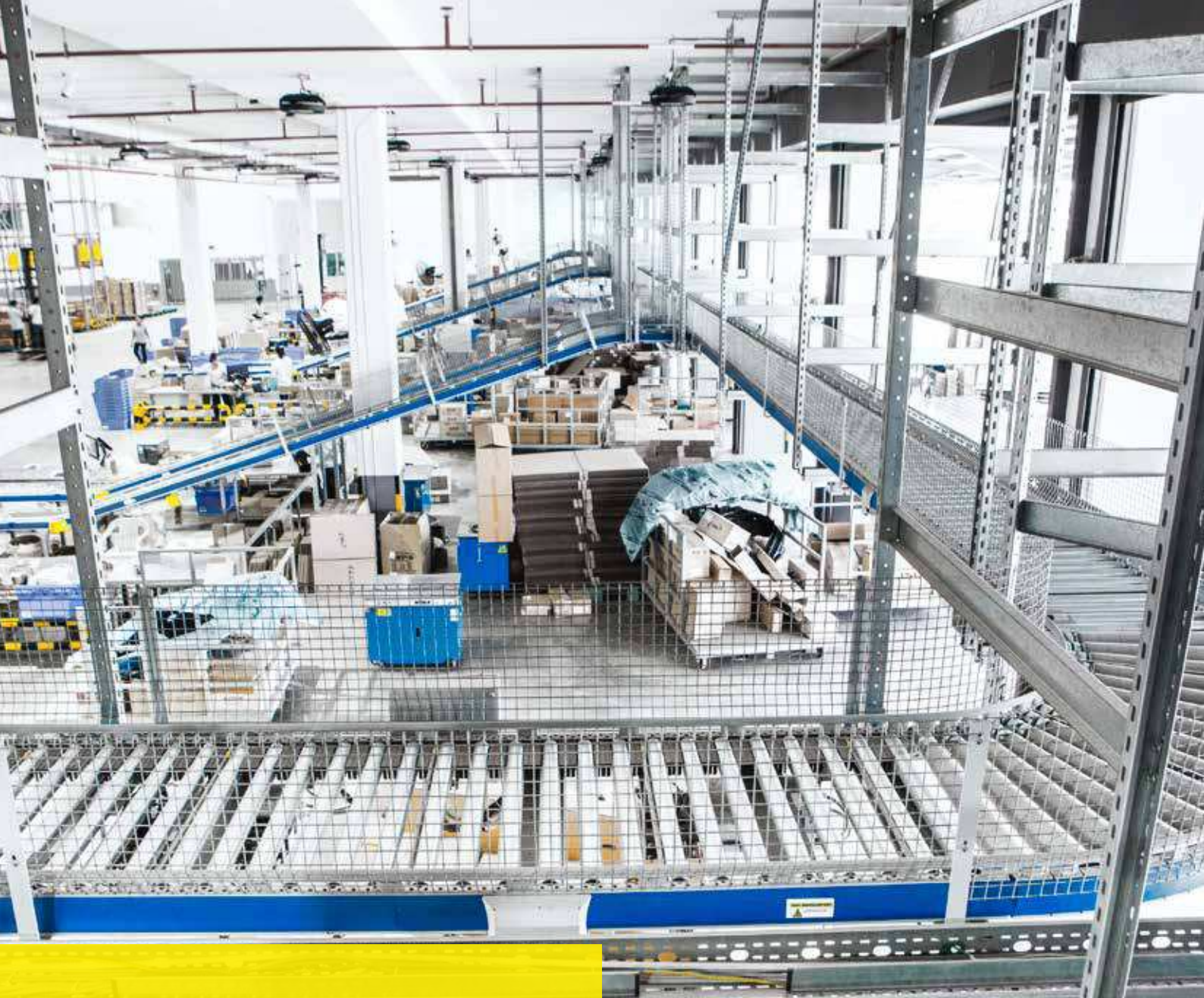
Carton and bin conveying systems and Work Stations
