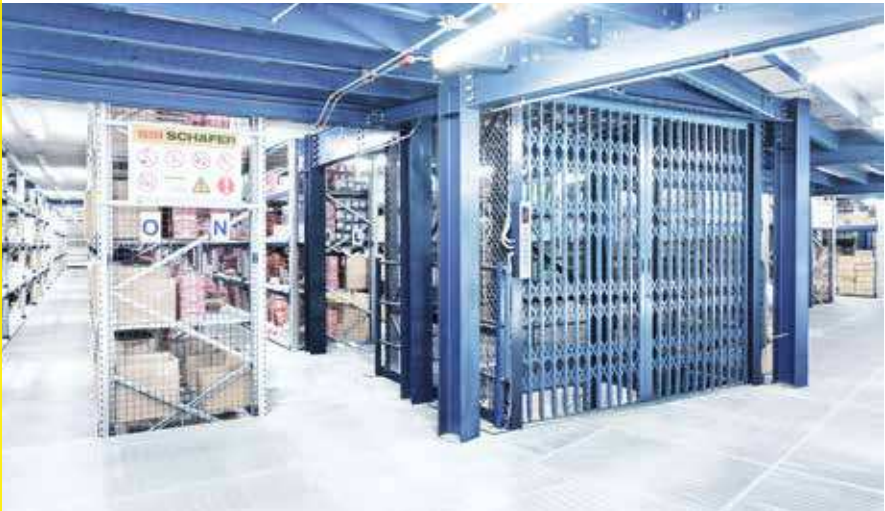
Goods lift integrated into platform system for access to all floors
